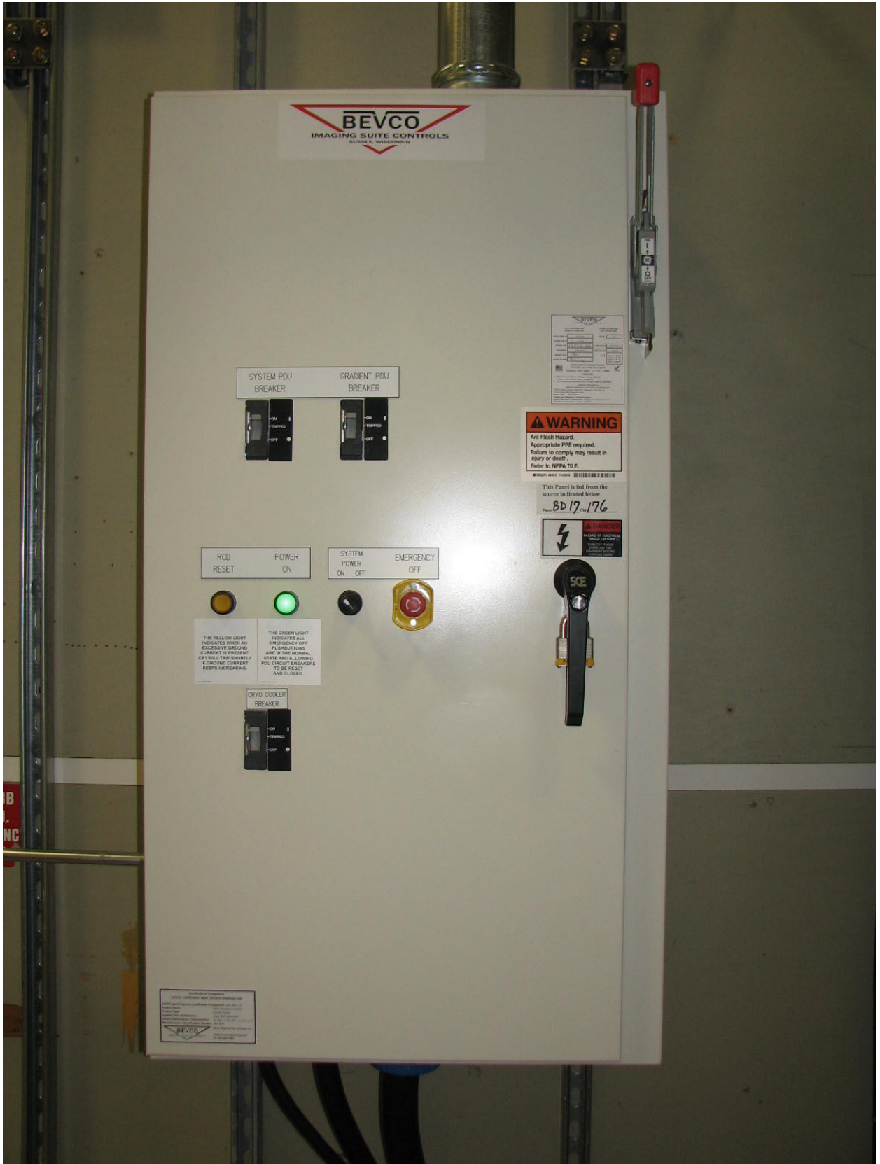
Figure 2-1 Main Disconnect Panel (MDP)
