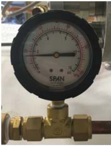
Figure 3-11 Magnet analog pressure gauge
