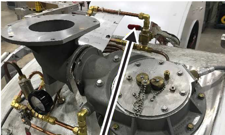
Figure 3-12 V3 valve in the closed position
