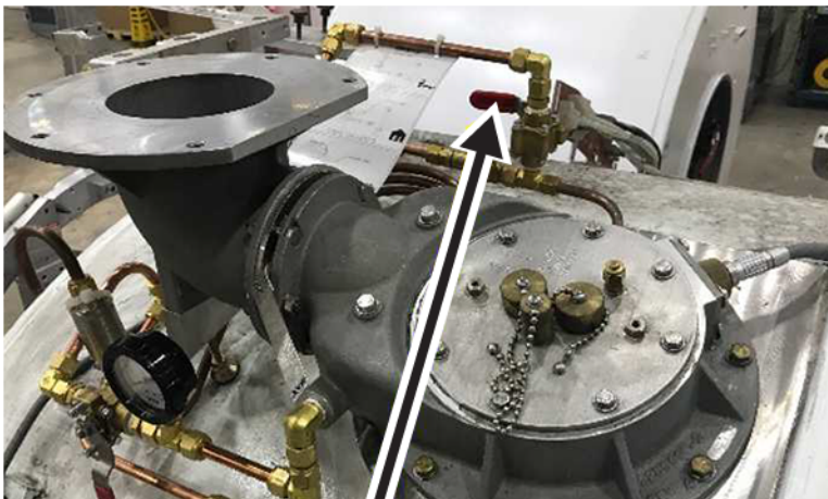
Figure 3-10 V3 valve in the closed position
