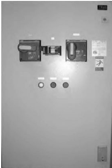
Figure 3-1 Main Disconnect Panel (MDP)
