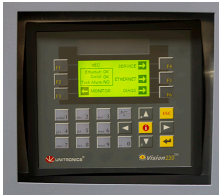
Figure 2-12 PLC signal box
