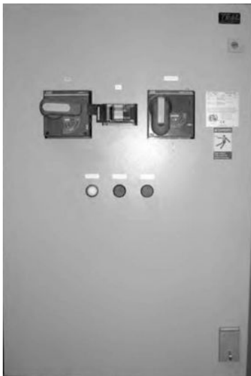
Figure 2-9 Main Disconnect Panel (MDP)
